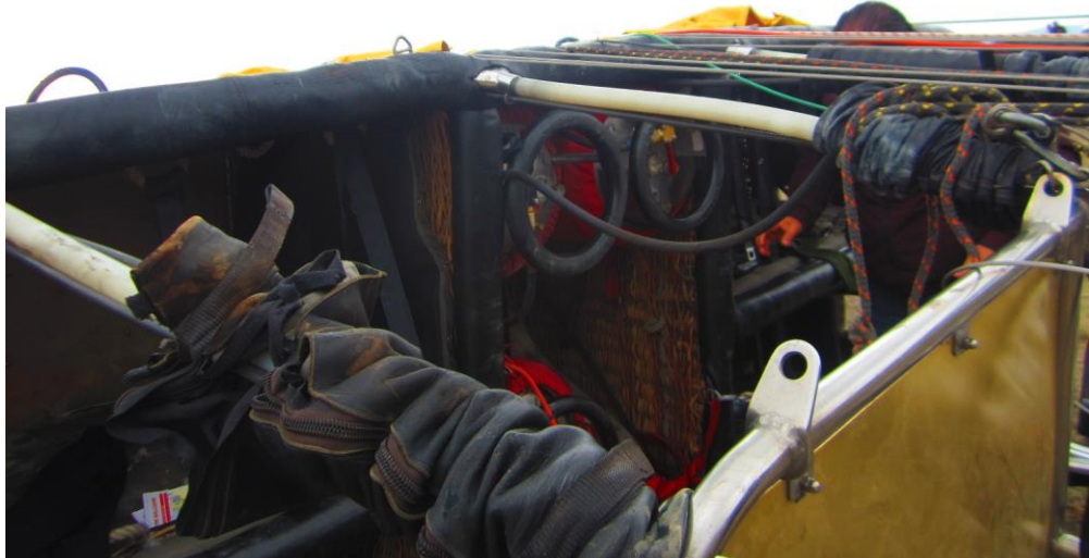
Picture-6: Burner Frame Housing Damage
